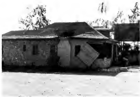
Photo 10. Unreinforced chimney which fell through roof of dwelling in San Fernando.
